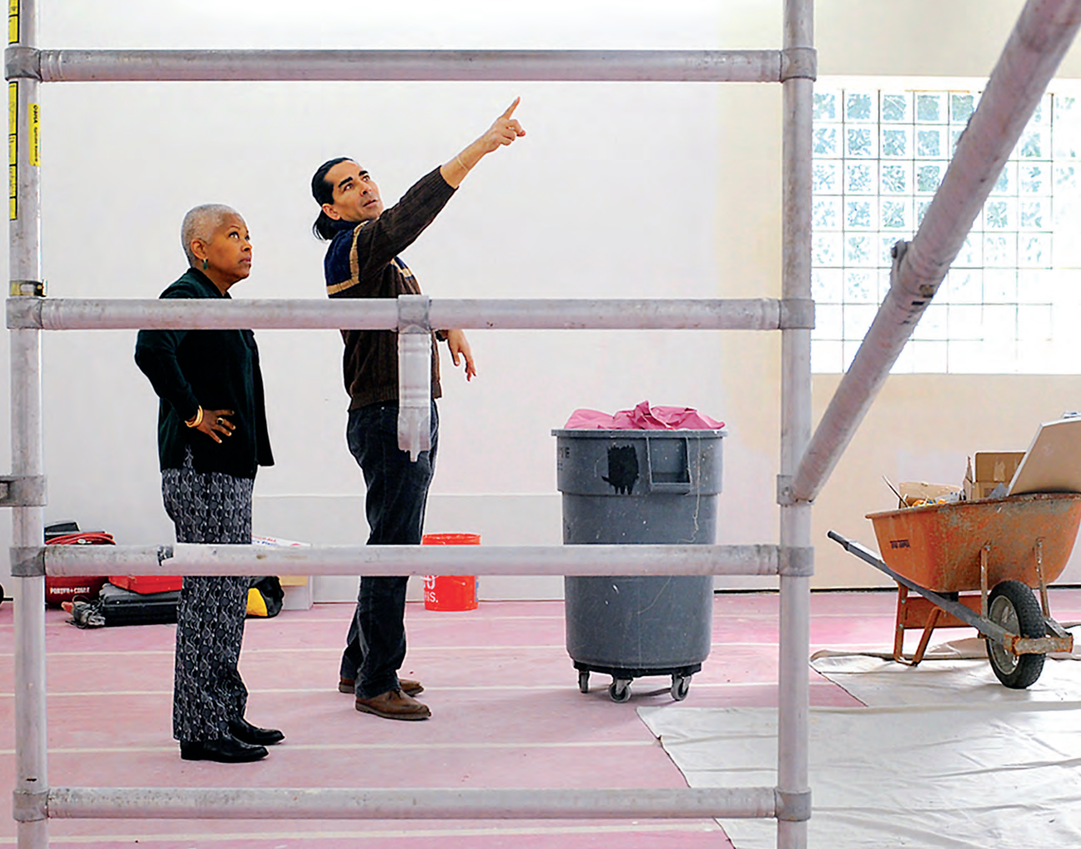
Art + Practice co-founders Eileen Harris Norton and Art + Practice Executive Director Allan DiCastro check on construction of the Exhibition Space. Photo by Christina House-Skalij.
